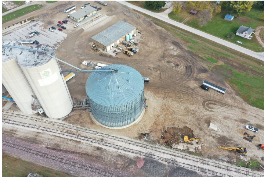
Pro Cooperative will be building a new 800,000-bushel bin and with the accessories south of the existing bins at the Graettinger location.
