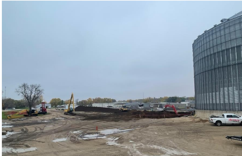
Dirt work started on October 25, 2023. The projected completion date of the project is August of 2024.
