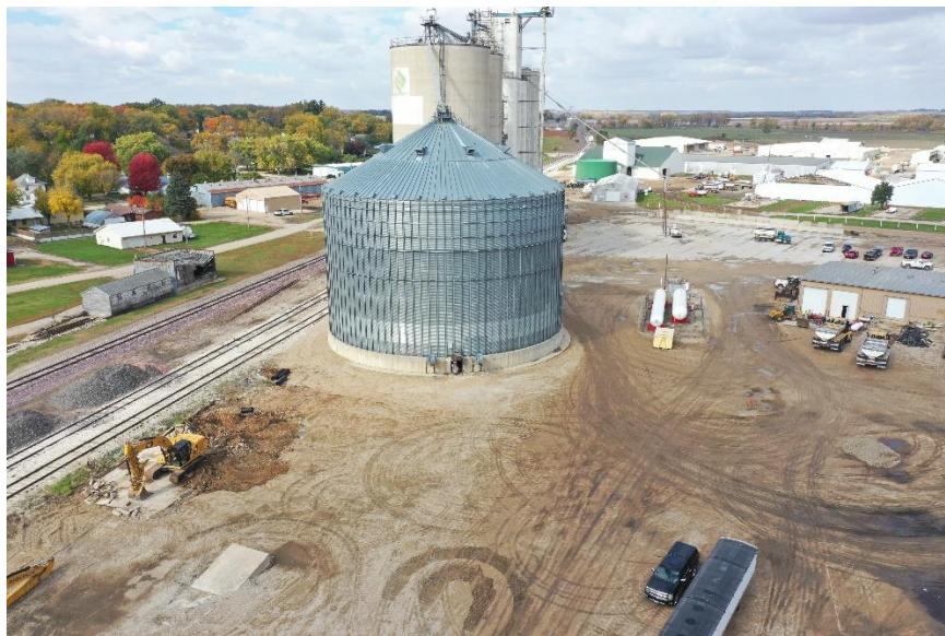
The new bin will be 105 feet in diameter and will also have a new 25,000 bushel per hour pit and leg added to the location.
